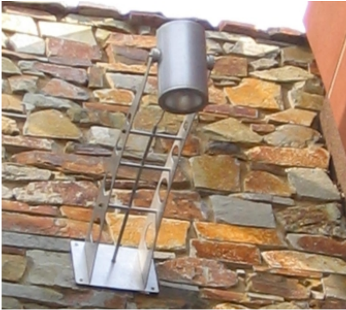
Beam downlighter 70W MH with special bracket and wall mounted pole.
