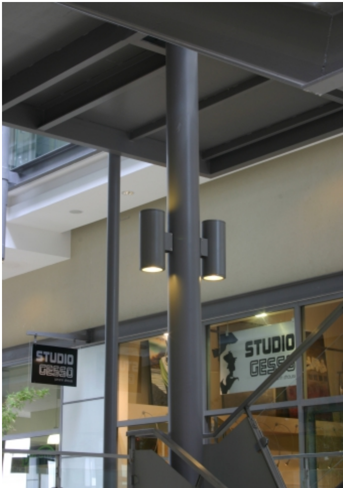
Beam up/down lighters c/w 20W Energy saver lamps
