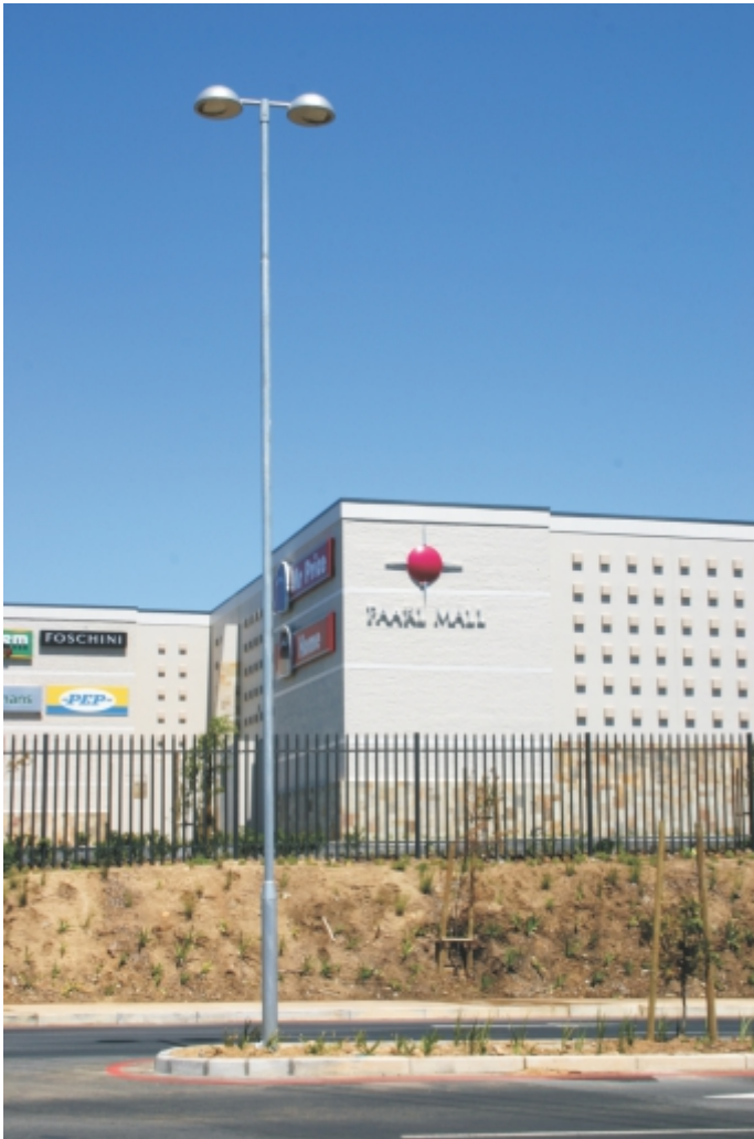
Double Sun Luminaires c/w 250W MH on 9m pole
