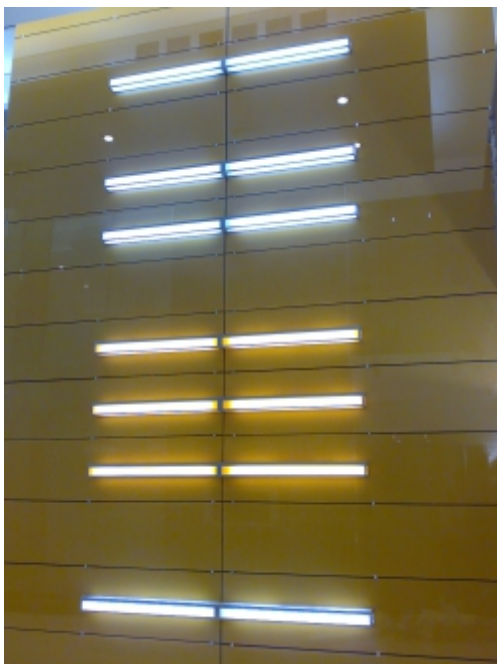
1.2m long special wall brackets with coloured perspex complete with 2 x 28W lamp & ECG
